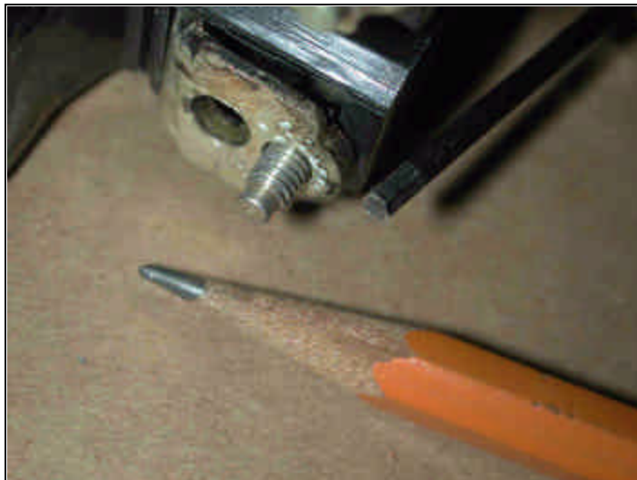
FIGURE 7 - ONE LOAD-SIDE CONTACT AND ITS 8-32 CLAMPING SCREW, ON THE FPE 100-AMP MAIN BREAKER OF FIG. 6. THE SCREW-HEAD TAKES A 3/32" ALLEN WRENCH, WHICH IS ONLY SLIGHTLY LARGER THAN THE LEAD OF THE #2 PENCIL. (The larger hole provides clearance for the screw protruding from the stab contact plate)
