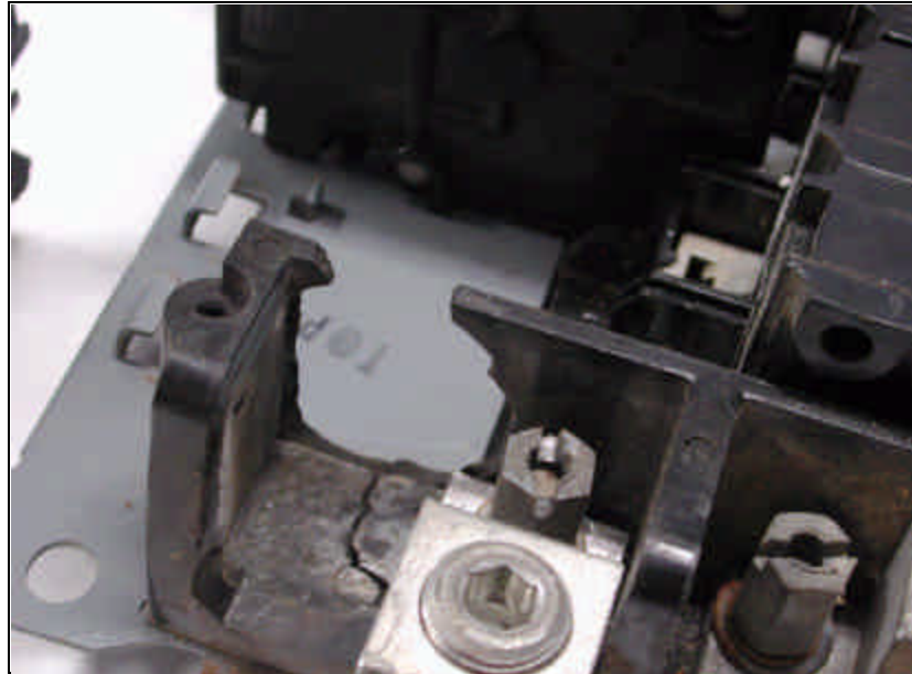
FIGURE 10 - THE DAMAGE TO THE INSULATING STRUCTURE OF THE PANEL (FIG. 8) IS MORE CLEARLY VISIBLE WITH THE BREAKER REMOVED.
