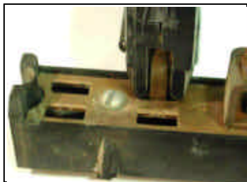
A. Copper buss bar with punched openings.
