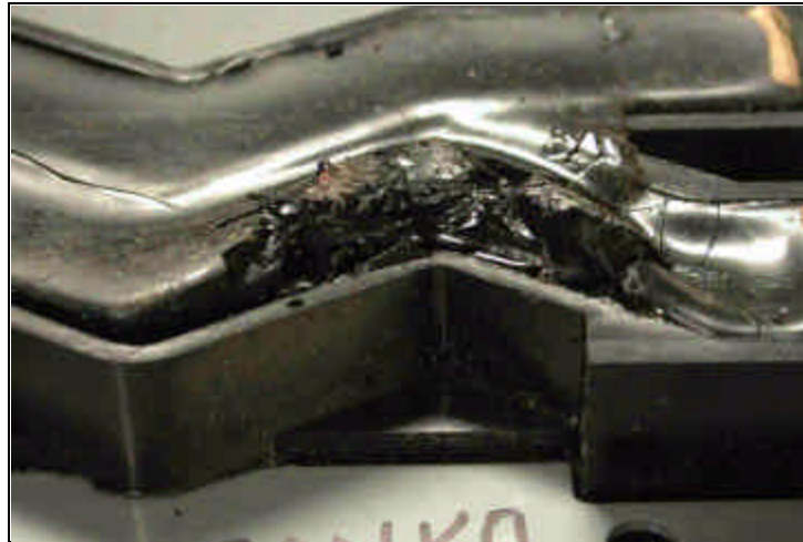
FIGURE 3 - OVERHEATING AT THE CONTACT BETWEEN THE BUSSBAR AND THE STAB SOCKET ASSEMBLY CAUSED THIS DAMAGE TO THE INSULATION. (This view is of the backside of the panel. The damage cannot not be seen unless the panel is taken out of the enclosure.)
